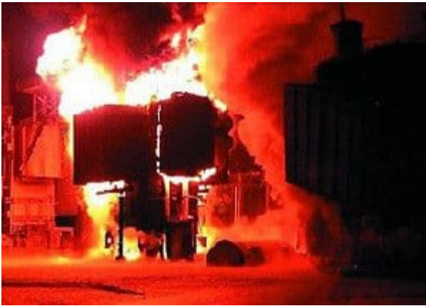
Transformer fire explosion
