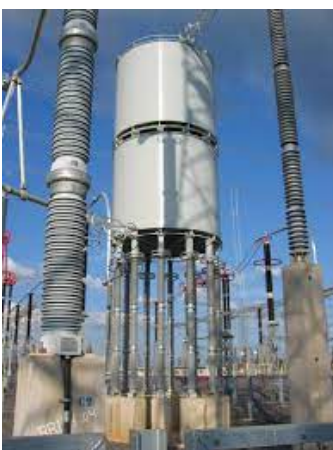
Fault current limiter
