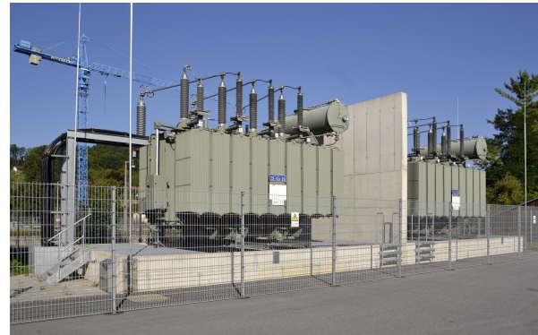
Transformer fire wall
