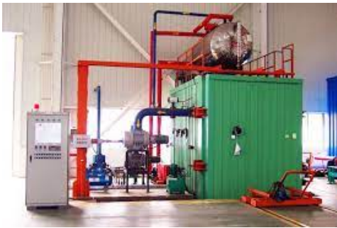
Vapor phase drying plant
