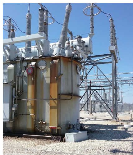
Leaks in transformer should be rectified at early stage
