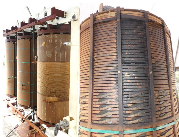
Internal inspection of transformer winding shows inter-turn fault
