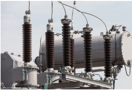
Mechanical forces can destroy transformer bushing
