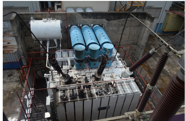
Bushing failure of generator transformer
