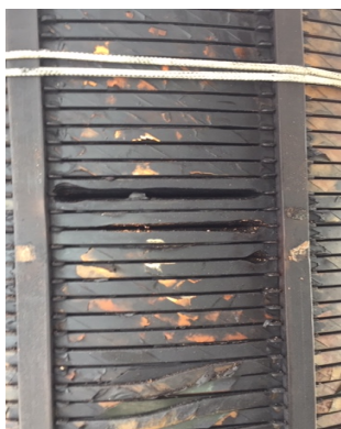
Winding failure due to short circuit between turn conductors
