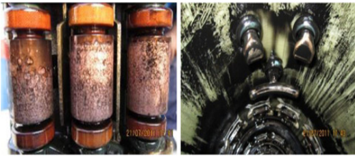
Surface erosion with pitted mark and coking of roller contact (left) and deposited of carbon on OLTC cylinder (right)
