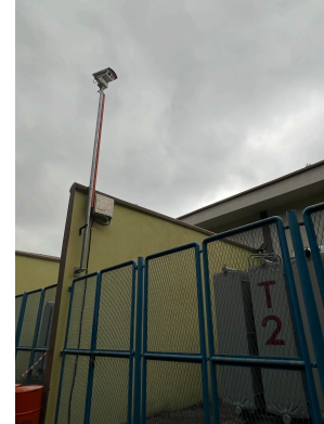
Online physical and infrared thermal inspection
